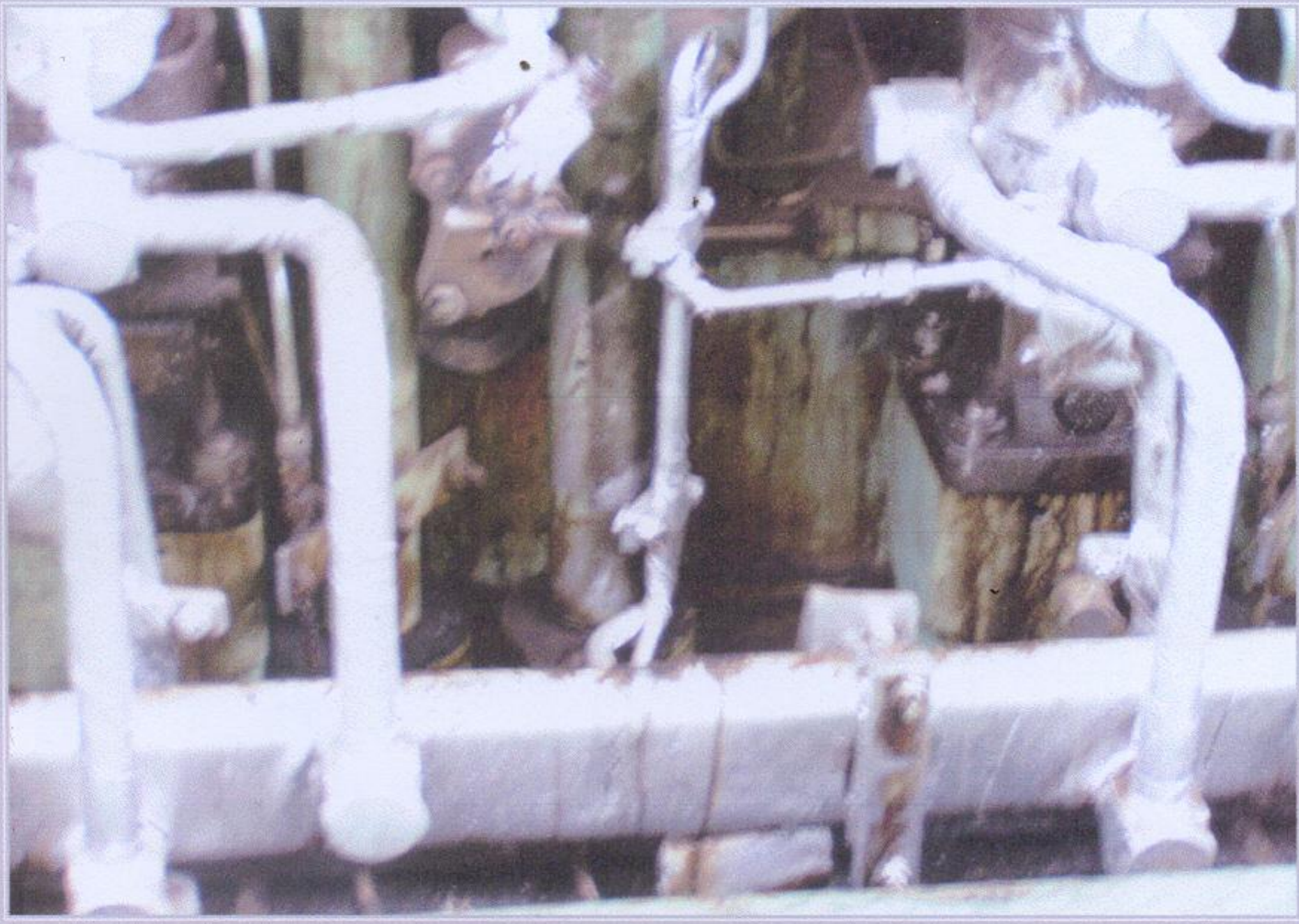
General Poor Condition of Engine Crankcase
