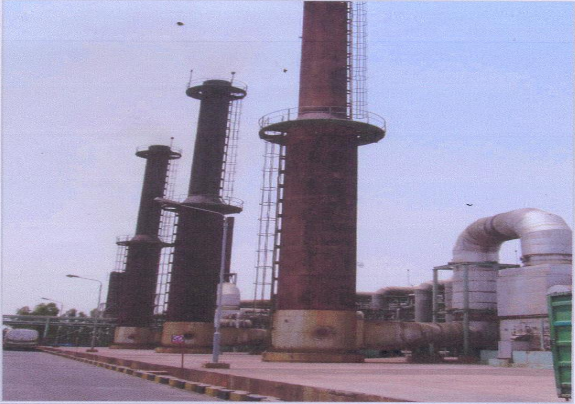
Rust Staining on Exhaust Stacks
