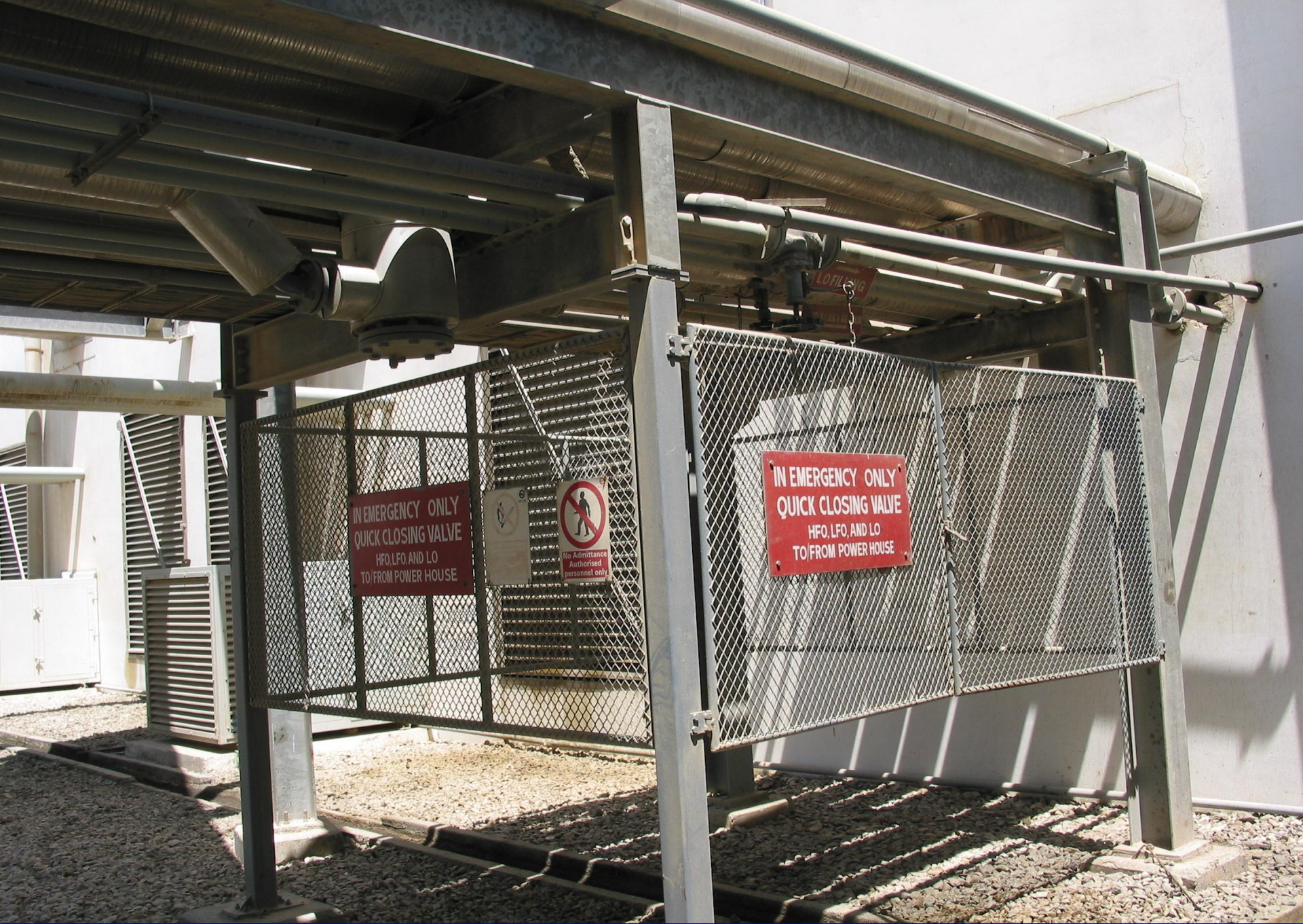
Fuel Oil Shut Off Valve
