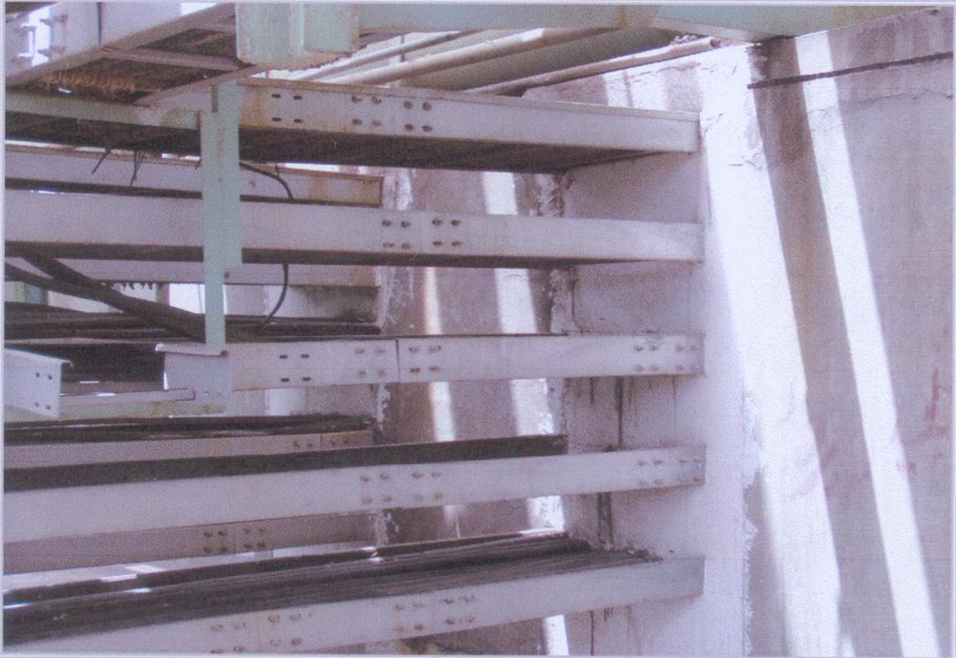
Effective Fire-Stopping on Cable Tray Penetration through external wall of Engine room above Ground level
