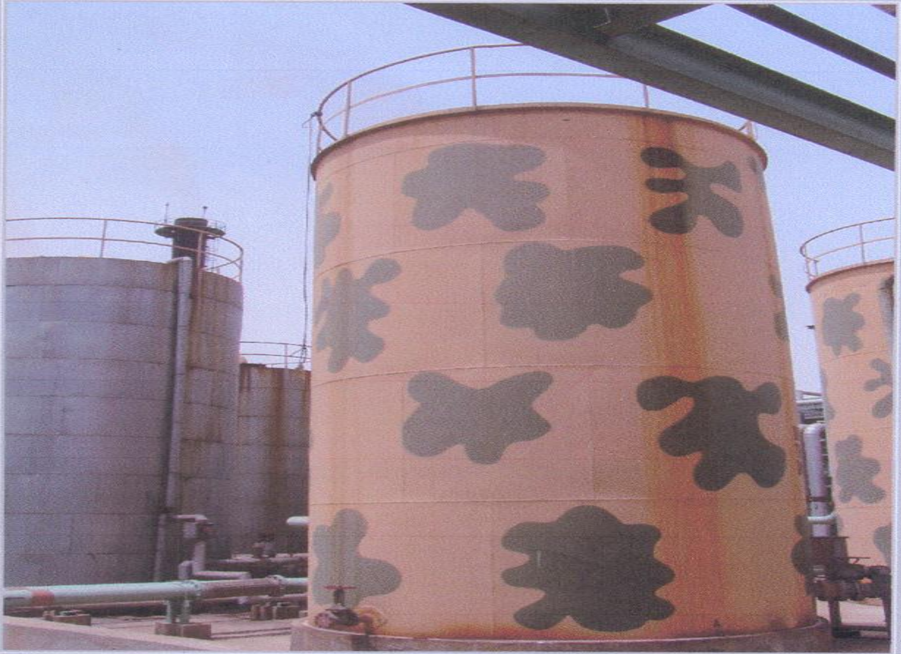
Rust Staining on Storage Tanks
