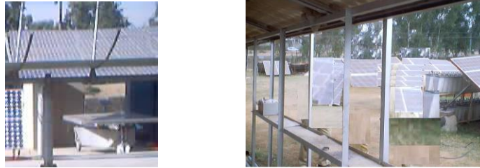
Fig 5. Several views of Solar Battery Charging Station in Rawalpindi
